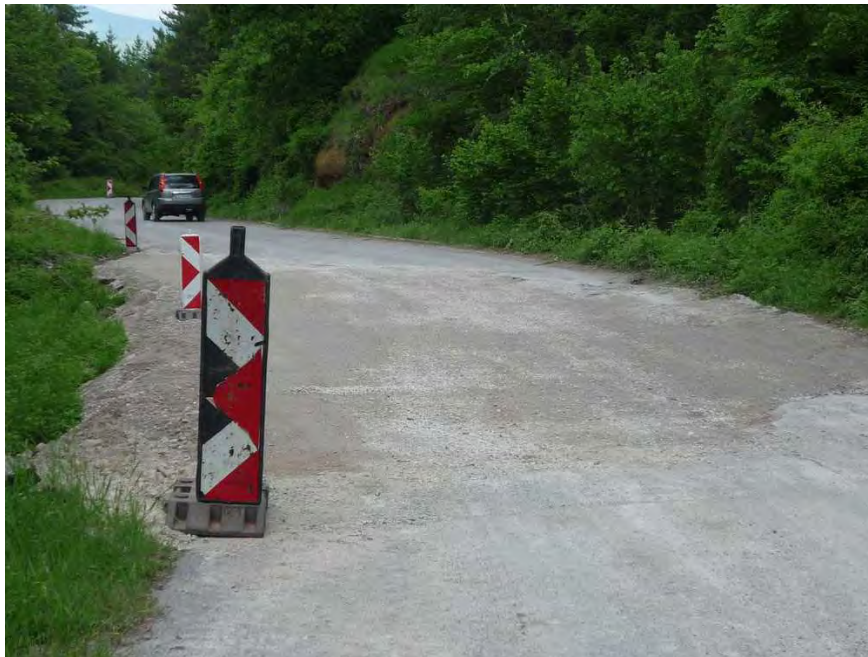
Figure 2.1. Landslide damaged section of road Rudartsi-Kladnitsa (GPS point 664).
