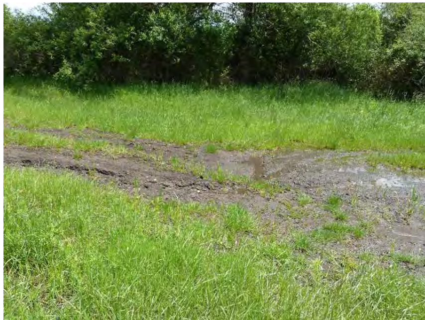
Photo 78. Small active alluvial fan along the line where cracks with displacement were observed.
